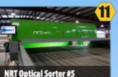
NRT Optical Sorter #5 Uses transmissive technology to recover PET plastics
