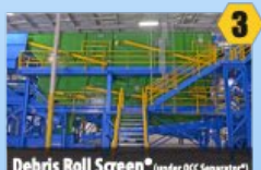
Debris Roll Screen* (under OCC Separator) Separates fines, including glass, from paper and containers
